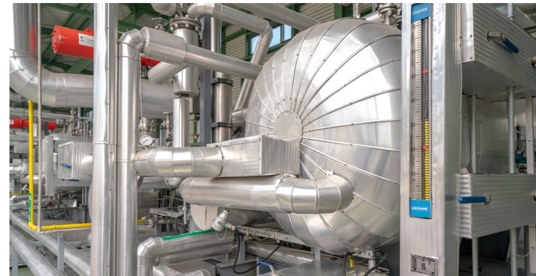
Hengli Petrochemical Refining flare gas transformation
