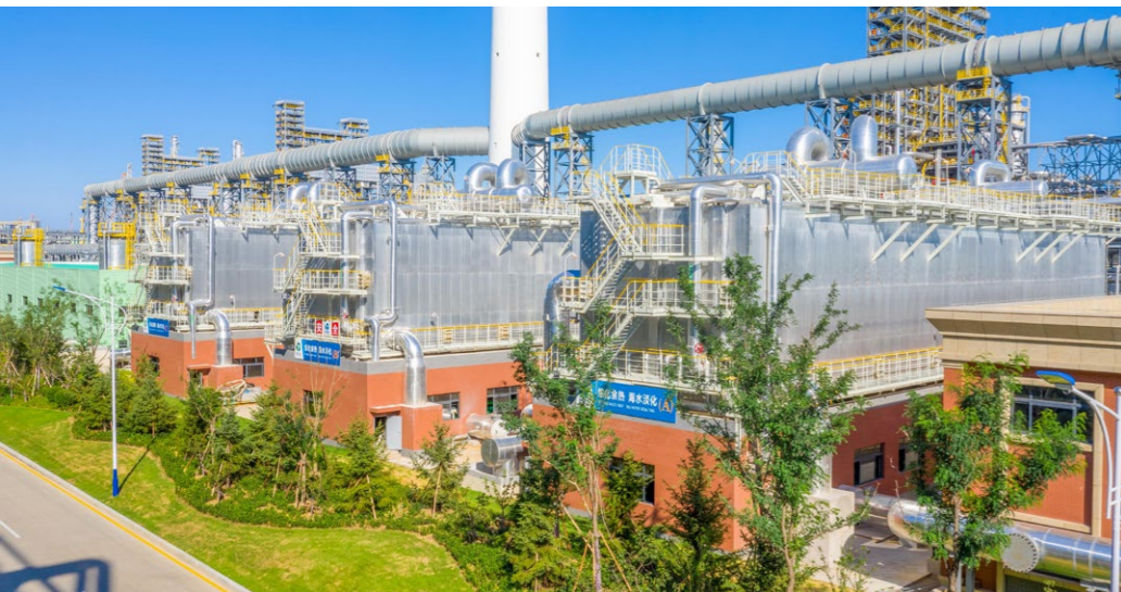
Hengli Petrochemical's seawater desalination facilities
